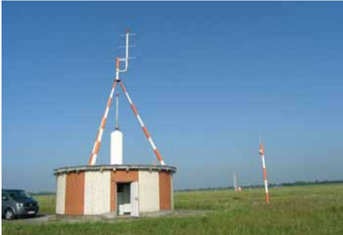
A GBAS system at Bremen airport
