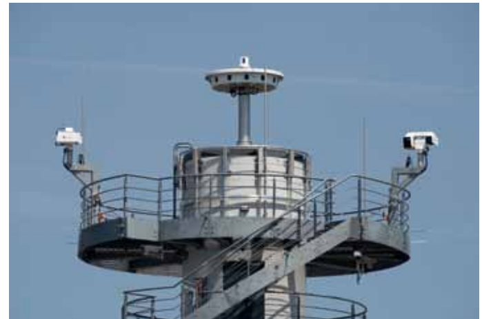
View onto the RTC (Remote Tower Control) camera tower of DFS in Saarbrücken
